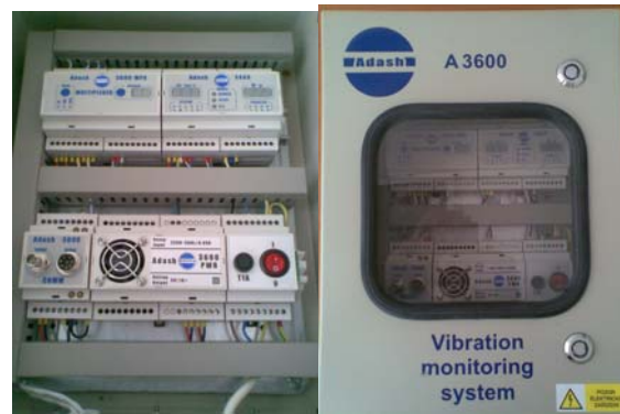
Fig. 2. Vibration monitoring system ADASH 3600
