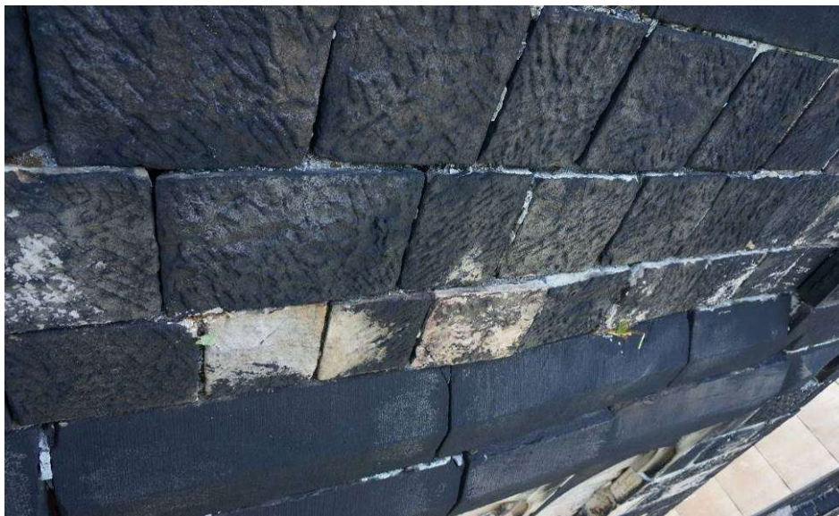
Fig. 14. North tower. Loss in joints, cracks in stone works, bumps in masonry units and the cornice
