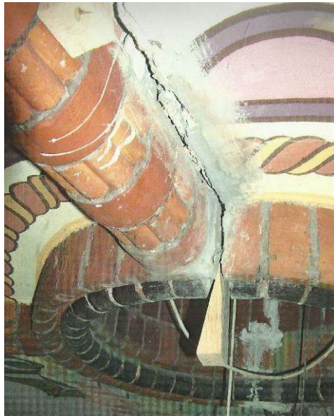
Fig. 9. Damaged area near the vault ribs and wood wedges driven in the place of cracking (2003)
