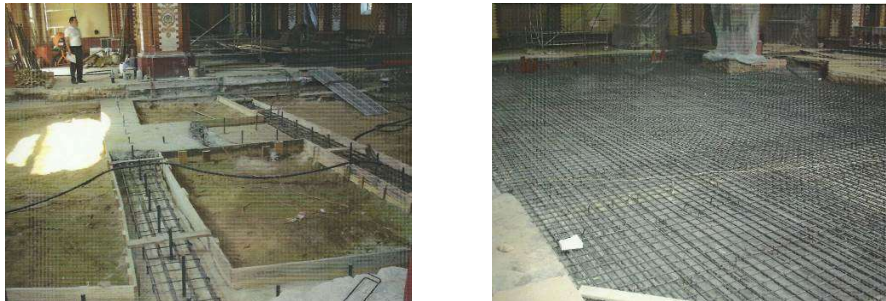
Fig. 5. Strengthening performed in the years 1986-1987: internal tie rods (left) and reinforcement of reinforced concrete slab (right)
