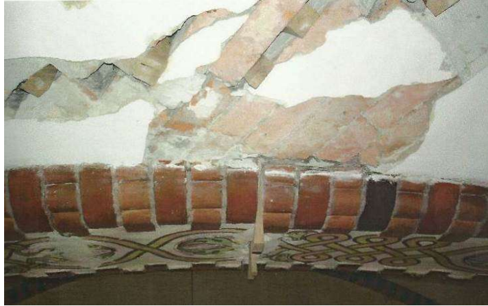
Fig. 8. Damage to the arch and wood wedges driven in the place of cracking (2003)
