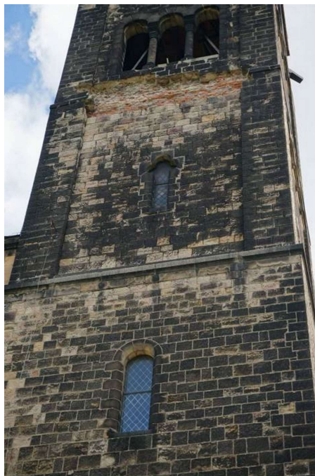
Fig. 11. View of damaged west elevation of the south tower
