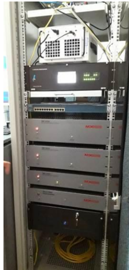
Figure 2. Rack of R-Mode equipment at the top
