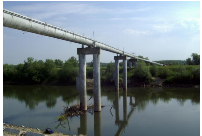
Fig. 1. A typical above-ground overpass of a long-operated gas pipeline in the Carpathian region.
