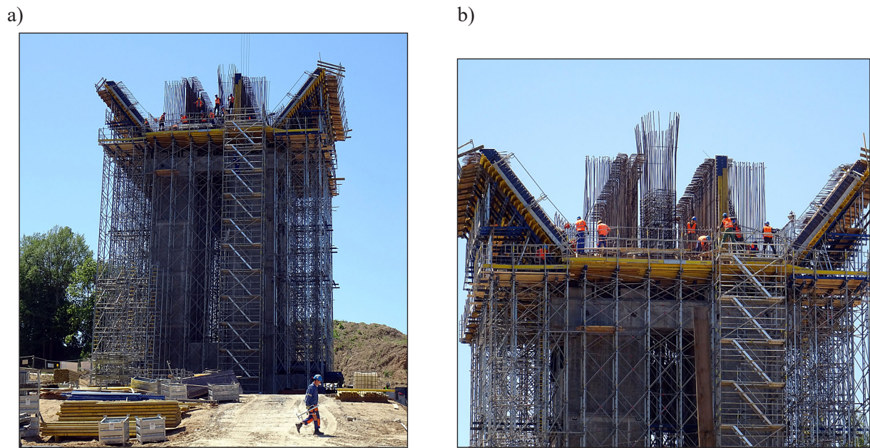
Fig. 4. First section on stationary scaffold (a), view of the deck section (b)
