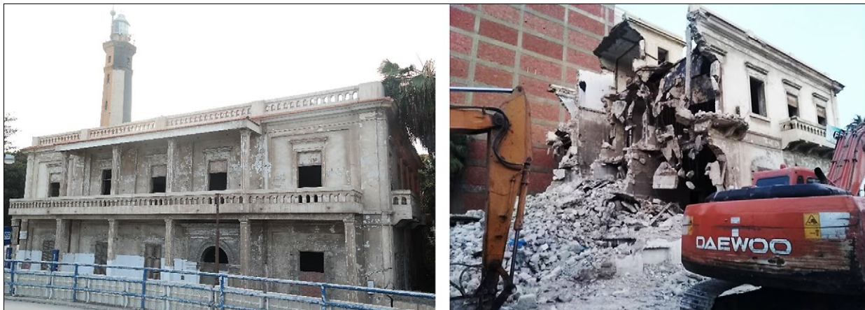
Fig. 4. Left: The American embassy in Port Said. Source: researcher. Right: The demolition in 2018. Source: researcher.
