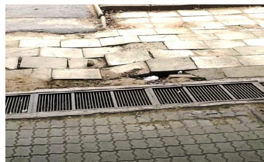
Fig. 2. Damaged sidewalk surface. Source: own photograph
