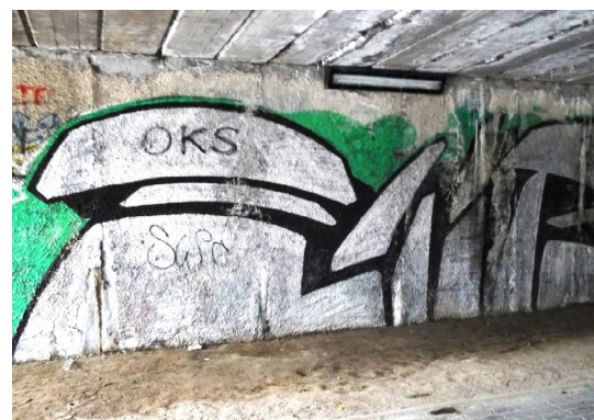
Fig. 3. Graffiti on the walls of the underground walkway. Source: own photograph
