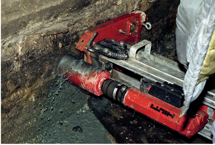
Fig. 3. Drilling the core no. 7 from the bottom plate of the foundation no. 1
