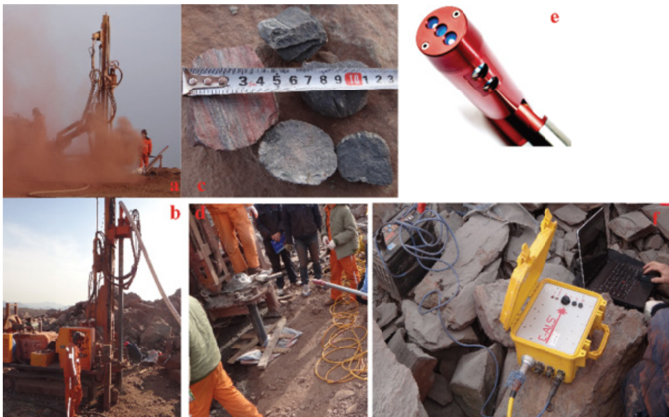
Fig. 11. The field testing site a: the dusty drilling site by using conventional drilling method; b: the clean drilling site by using RC-DTH air hammer drilling method; c: cores obtained by RC-DTH air hammer drilling method; d: preparation of detection after drilling by using RC-DTH air hammer drilling method; e: the detection unit of the cavity auto scanning system; f: scanning process by using the cavity auto scanning system
