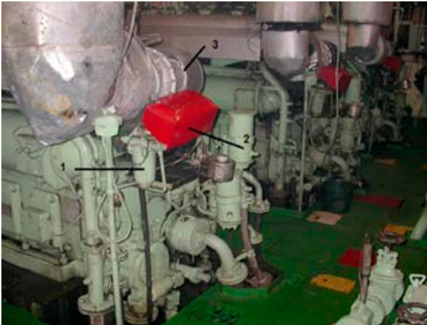
Figure 2. View of an auxiliary engine from side of the fuel filter on the ship from the series B-542: 1 – fuel filter, 2 – filter cover, 3 – turbocharger
