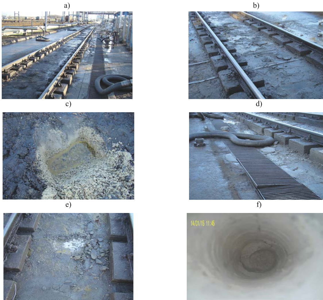
Fig. 3. Track with track bed: a) general view, b) damage to the main part of the track bed, c) open pit in the middle of the track between the rails, d) damage to the drainage channel, e) open pit - control hole, f) the interior of the control hole
