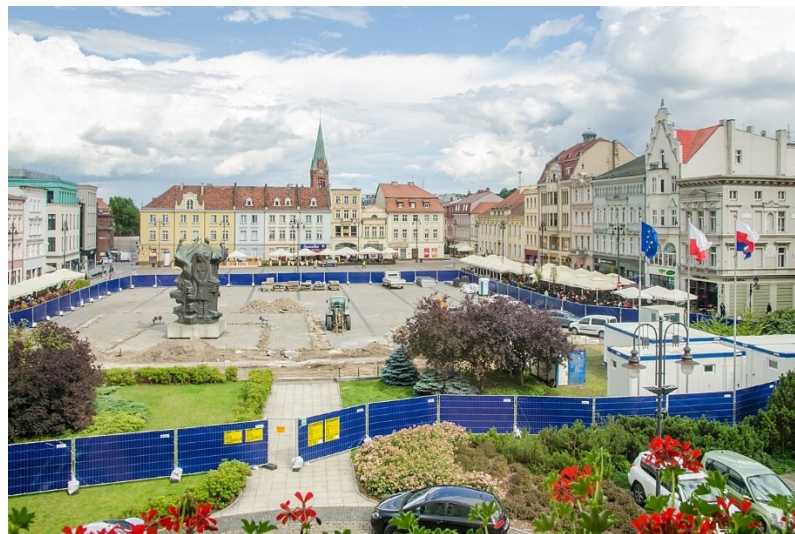
Figure 1. Revitalization works on the Old Market Square in Bydgoszcz. Source: Bydgoszcz w Budowie [Bydgoszcz under construction – Old Market Square] website, Beginning of revitalization, 22.10.2021.
