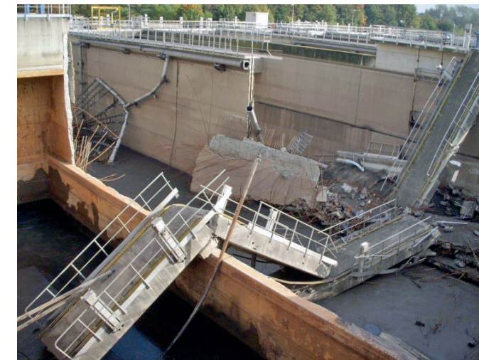
Fig. 8. Collapse of separation wall between full basin at down left, and emptied basin at right
