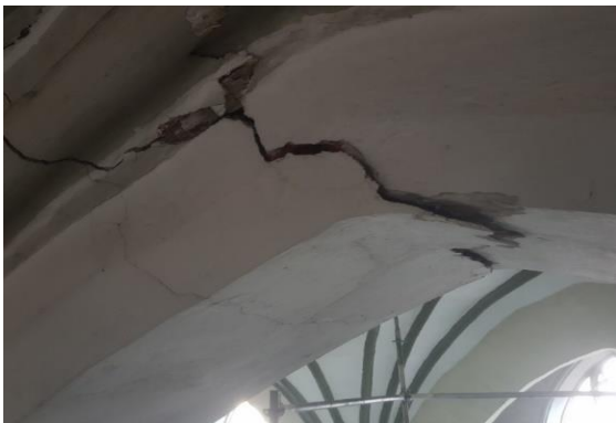
Photo 2. Damage to the arch between pillars 2 and 3 of the southern aisle of the Basilica of St. Nicholas in Gdańsk ( photo by T. Majewski )
