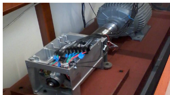
Fig. 5. View of the measurement set for investigation of the 5.5 kVA salient pole synchronous generator
