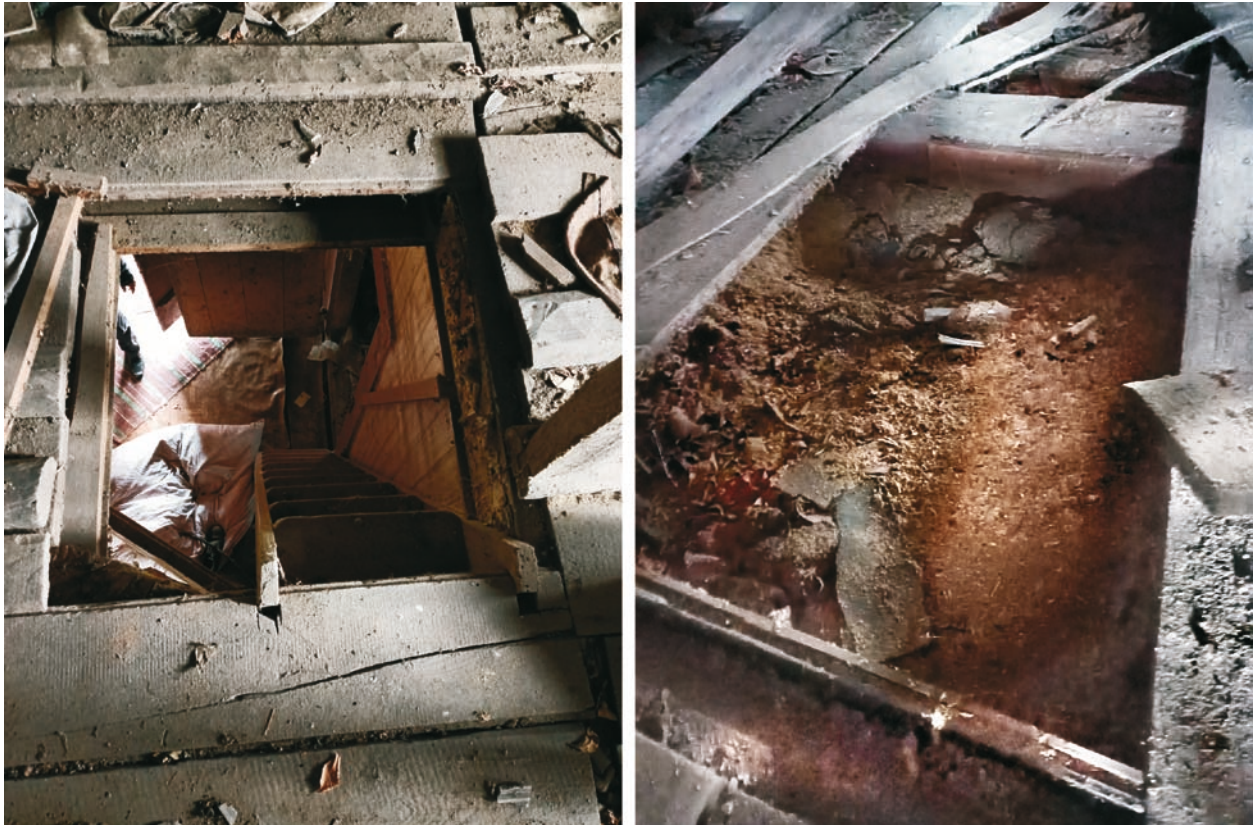
Fig. 11. Garret floor construction (a – ladder descending to the entrance hall; b – earthen insulation); source: the authors, 2021
