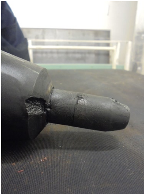
Fig. 3. High risk damage of FIV related to SECA fuel changeover, i.e. seating burnt out by combustion gas blow-by
