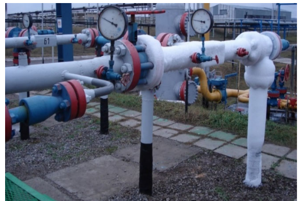
Fig. 2. General view of the piping at the gas pipeline inlet of the installation of disconnecting devices at the gas gathering station
