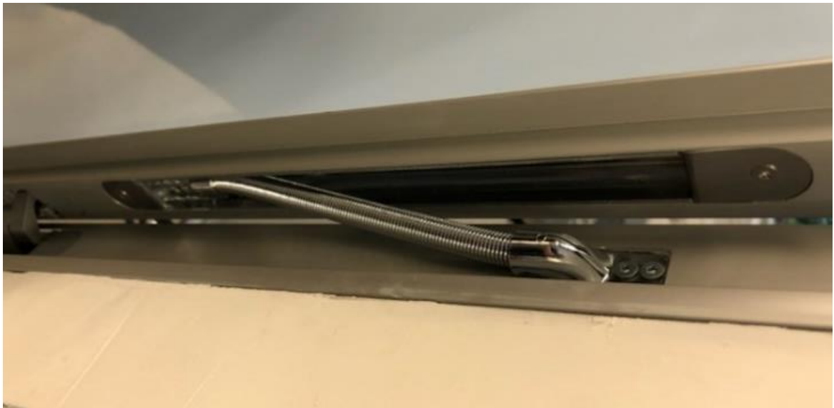
Fig. 13 Photo showing a cable gland placed in the door leaf and frame. Source: authors
