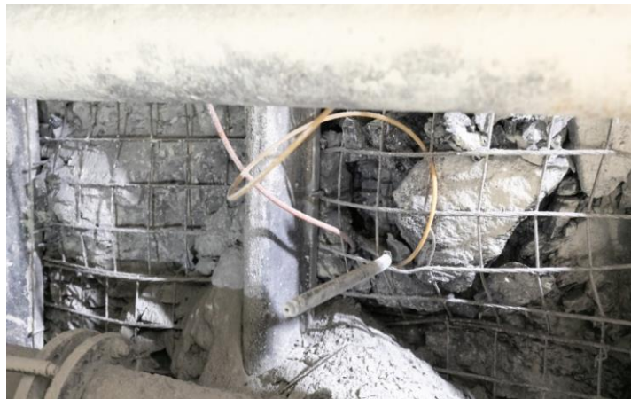
Fig. 5. Biaxial stressmeter installed in the wall of the excavation. Visible is the vent tube used for grouting the sensor in the rock.
