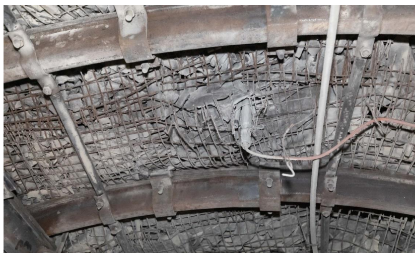
Fig. 11. Instrumented rock bolt installed in the roof of maingate PW-1. Visible is the end of the packer used for grouting.
