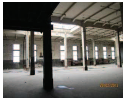
Fig. 23. Current situation inside cotton storage space of Makbas Eltarekk (Source: authors, 2012)
