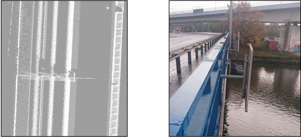
Figure 10. Visible elements in the extreme part of the span (left picture); identification was based on additional photographs (right picture)
