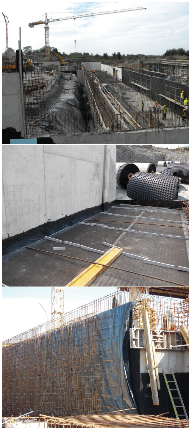
Figure 5. Installation of anti-vibration mats in segment A of the building: building-site overview; horizontal anti-vibration insulation; vertical anti-vibration insulation protected with foil
