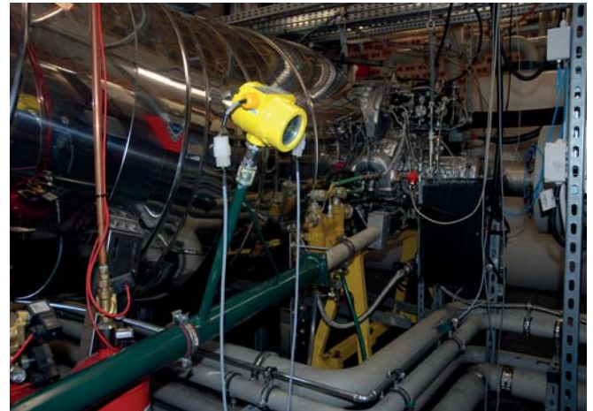
Photo 3. Measurement of extraction air parameters on the gas turbine test stand
