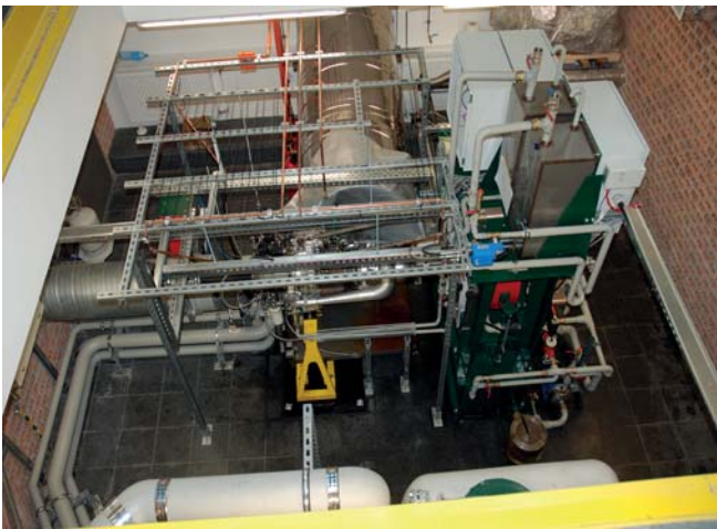
Photo 2. The test and didactic stand containing the two-shaft gas turbine
