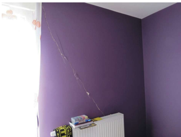
Fig 8. Cracks in the east outer cover wall on the first floor in the first segment (apartment number 1) (Praca ... 2016)
