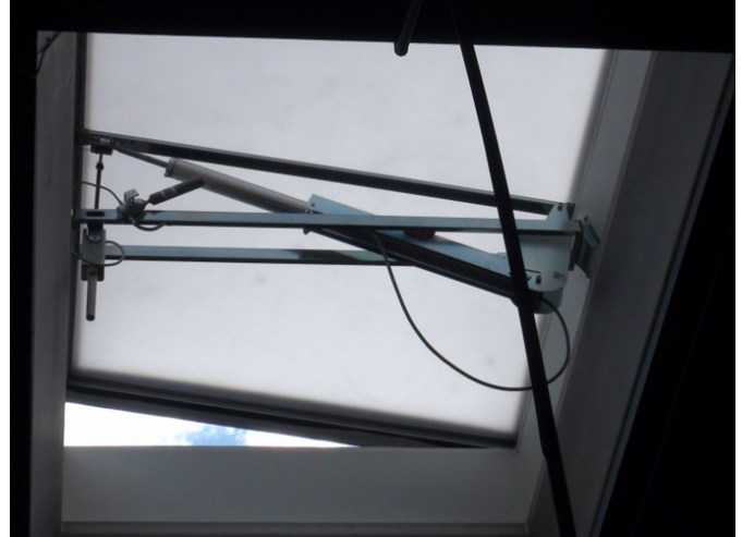
Fig. 2. Linear EMA with screw gear controlling the opening the smoke extraction flap located on the building's roof
