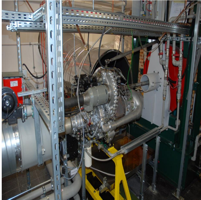
Img 1. View of a two-shaft gas turbine
