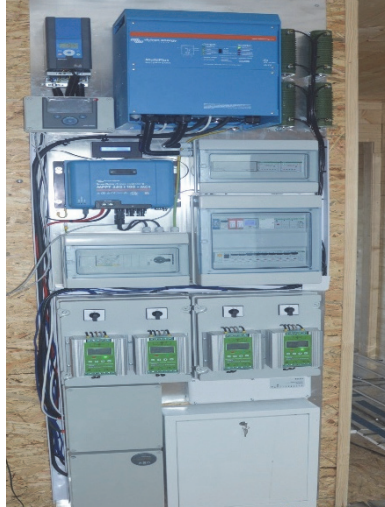
Fig. 8. General view of the WH hybrid power supply system
