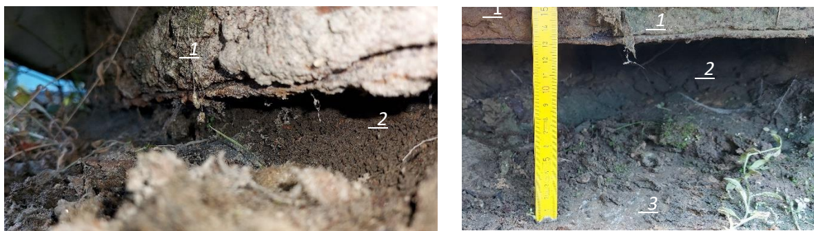
Figure 8. Sand foundation zone of the tank; 1 - steel bottom of the tank, 2 - washed sand from the ground, 3 - reinforced concrete slab
