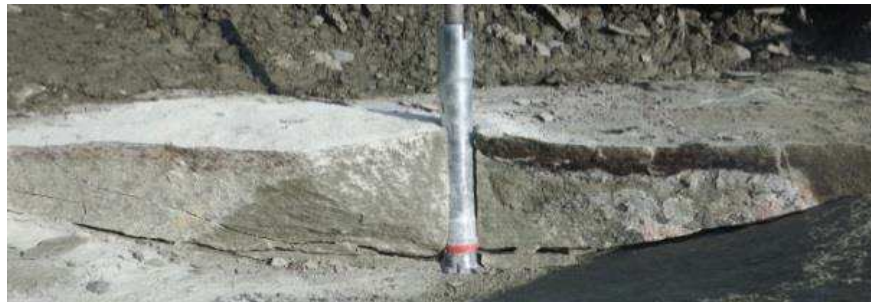
Fig. 15. Under-cutting bolt: method of the bolt fixation and range of loosening fracture propagation [20]
