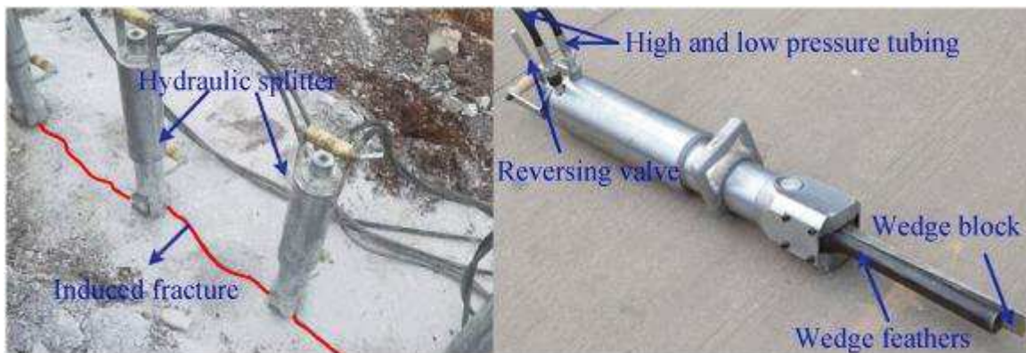
Fig. 8. Hydraulic splitter employed for the non-explosive fracturing of rock in engineering application [21]
