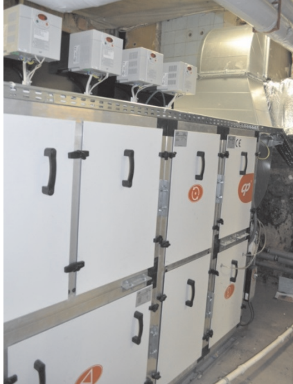
Fig. 2. Fragment of the ventilation central unit with a rotary exchanger for heat recuperation
