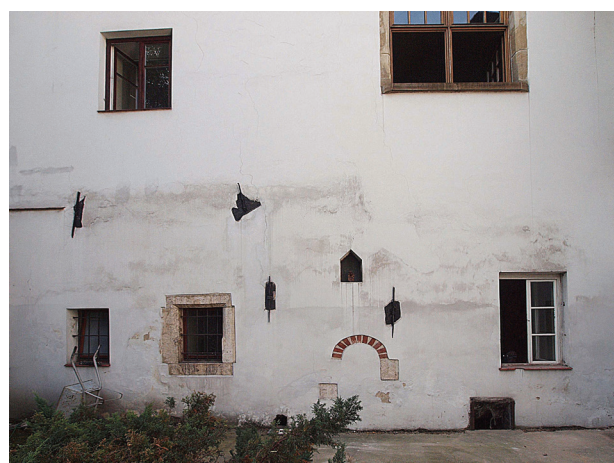
Fig. 3. Dominican priory in Krakow – the northern elevation of the eastern wing of monastery located at the 3 rd cloister, relics of the façade composition at the ground floor: portal with semicircular brick archivolt and windows, partly rebuilt (photo by A. Bojęś-Białasik)
