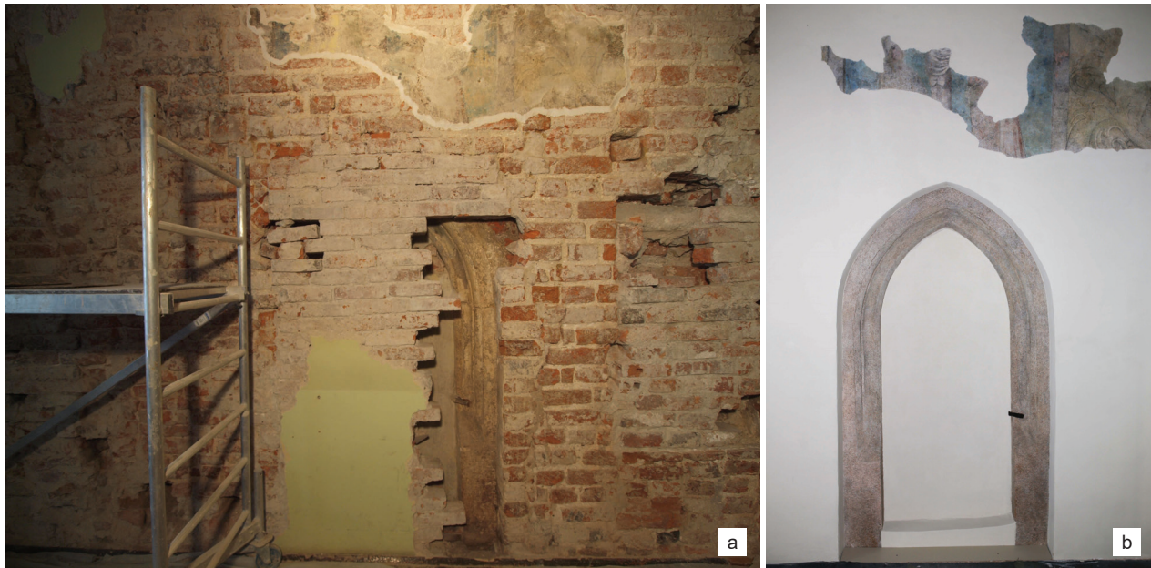
Fig. 6. Dominican priory in Krakow – the eastern wall with a brick covering and a fragment of polychrome above it (Crucifixion?): a) gothic portal while uncovering, b) gothic portal and polychrome after conservation work completion (photo by A. Luboń-Radwańska)
