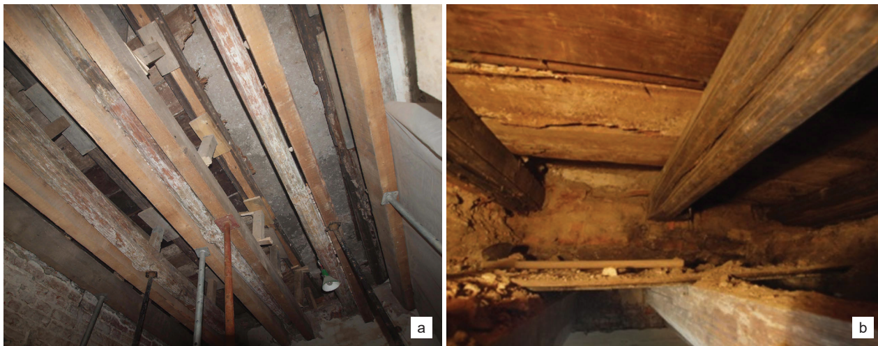
Fig. 8. Dominican priory in Krakow – wooden beam ceiling (“higher” one) – “technological”: a) both ceilings while exploring with intervention support, b) rubble charge filling the space between the ceilings (photo by A. Bojęs-Białasik)
