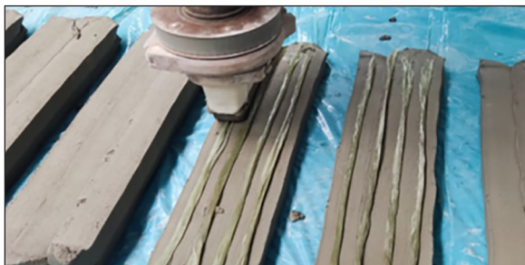
Figure 1. Printing the second layer of concrete (with a trapezoidal nozzle) of an automatically reinforced beam (sample no. 42RT)
