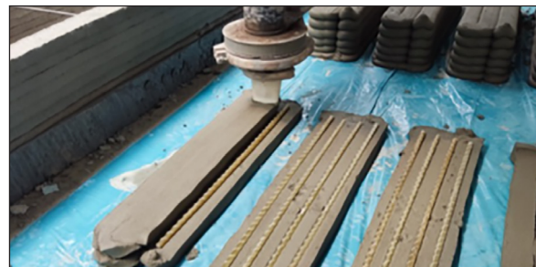
Figure 2. Printing the second layer of concrete beam (with a trapezoidal nozzle) in a conventional composite reinforced beam (sample no. 11KT)
