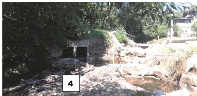
Fig. 2. Damages in the Kacza river estuary area in Gdynia Orłowo as a result of the freshet in July 2016 (photos No. 1, 2, 3 – washout of sea-shore belt below Orłowska street bridge, photo No. 4 - breach in road embankment of Zapotoczna street. Location of subsequent shots – see Fig. 1. ( acc. this author's archive)
