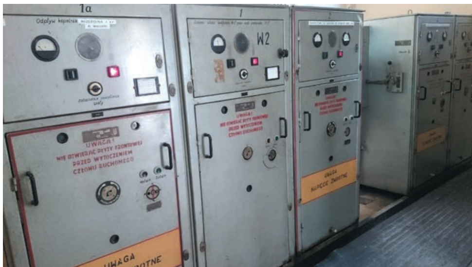
Fig. 2. Field distribution station type RSK-6 of the 3 kV MV “Wilson” switchgear
