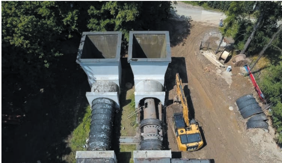
Fig. 1. Main ventilation fans for “Wilson” shaft
