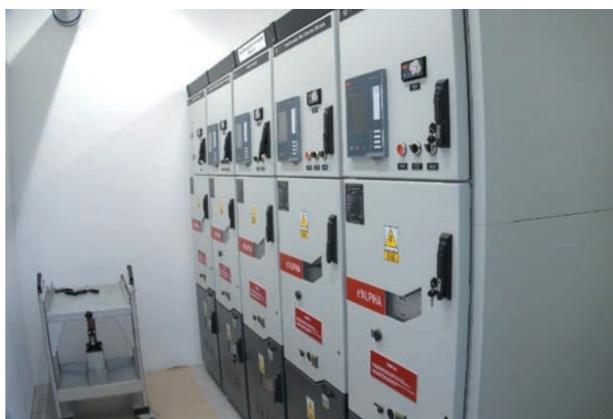
Fig. 5. e 2 ALPHA distribution cells of the 3 kV MV “Wilson” switchgear
