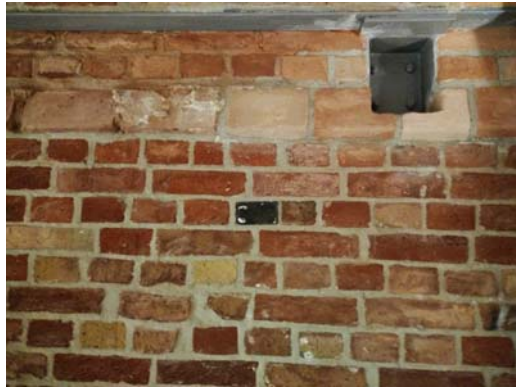
Fig. 14. Using mortar painted into color of wall instead of bricks in unusual size. Source: K. Wierzbicki, October 2016
