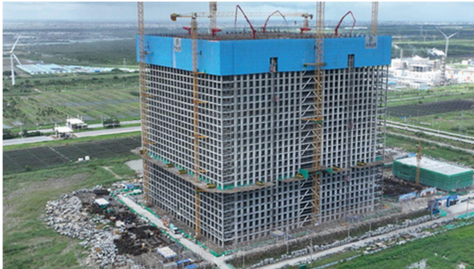
Fig. 3. Energy storage system in, China under construction [Image: Energy Vault, Business Wire ]
