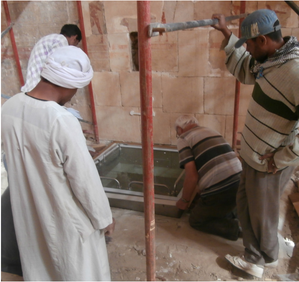
Fig. 7. Installation of a manhole to the tomb of members of the royal family from the 23 rd –25 th dynasties (S.7A/82), 2013 (photo by T. Dziedzic)
