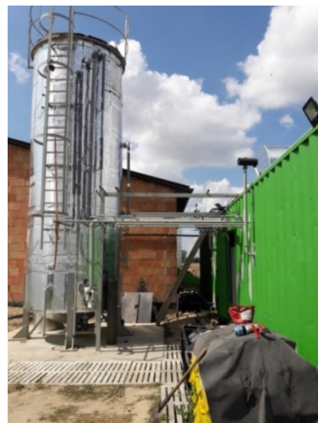
Photo 1. Pilot installation – examples of techniques of the anaerobic fermentation of waste – mono-substrate reactor (phot. G. Wałowski)
