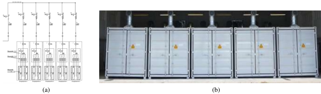
Fig. 3. A 5 MW/1 h BES in test: (a) electric schema of the five strings; (b) front view of the BES
