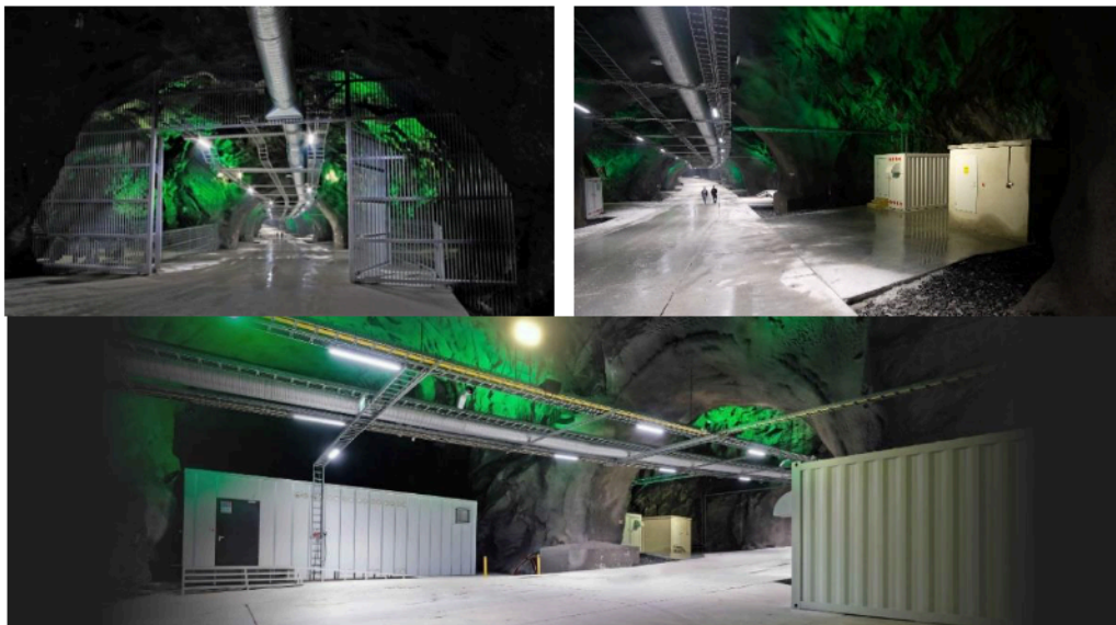
Fig. 15. The most energy-efficient server room in Europe located in the Norwegian Lefdal olivine mine 150 m underground [18]
