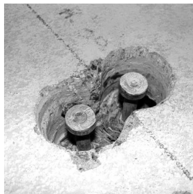
Fig. 3. Damage of the connection
