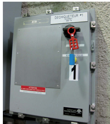
Figure 1. Individual lock applied on an electric isolating device.
