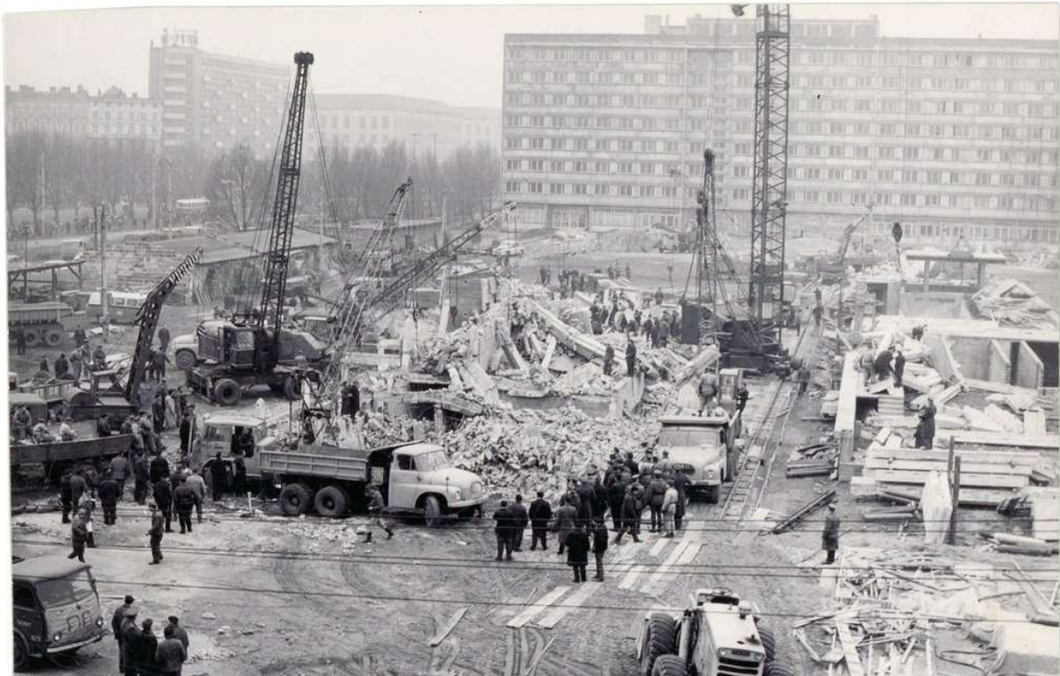
Photo 1. Construction disaster during the construction of the building of the Land Reclamation Department for the Higher School of Agriculture in Wrocław (1966) Source:
