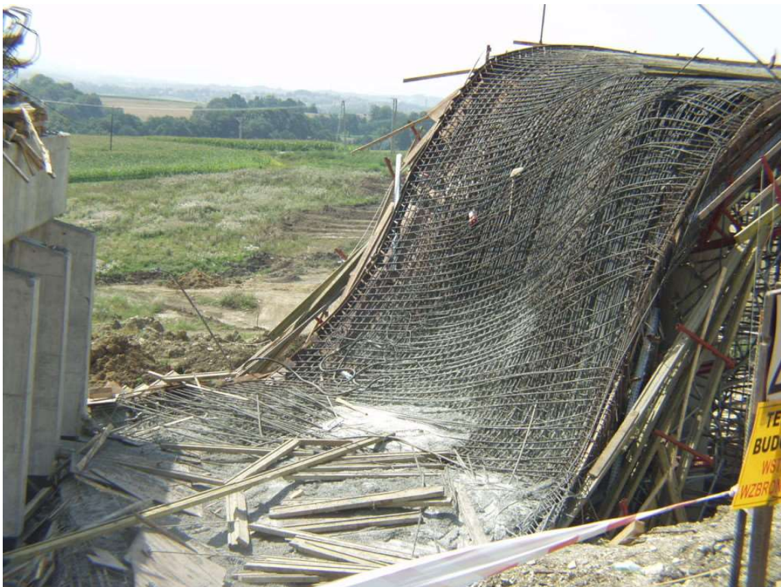
Photo 8. Disaster of the viaduct built on the national road No. 1 in the village of Ogradzona, 4.08. 2003, Source: https://nemu.com.pl/case-studies/zawalenie-sie-konstrukcji-wiaduktu/
