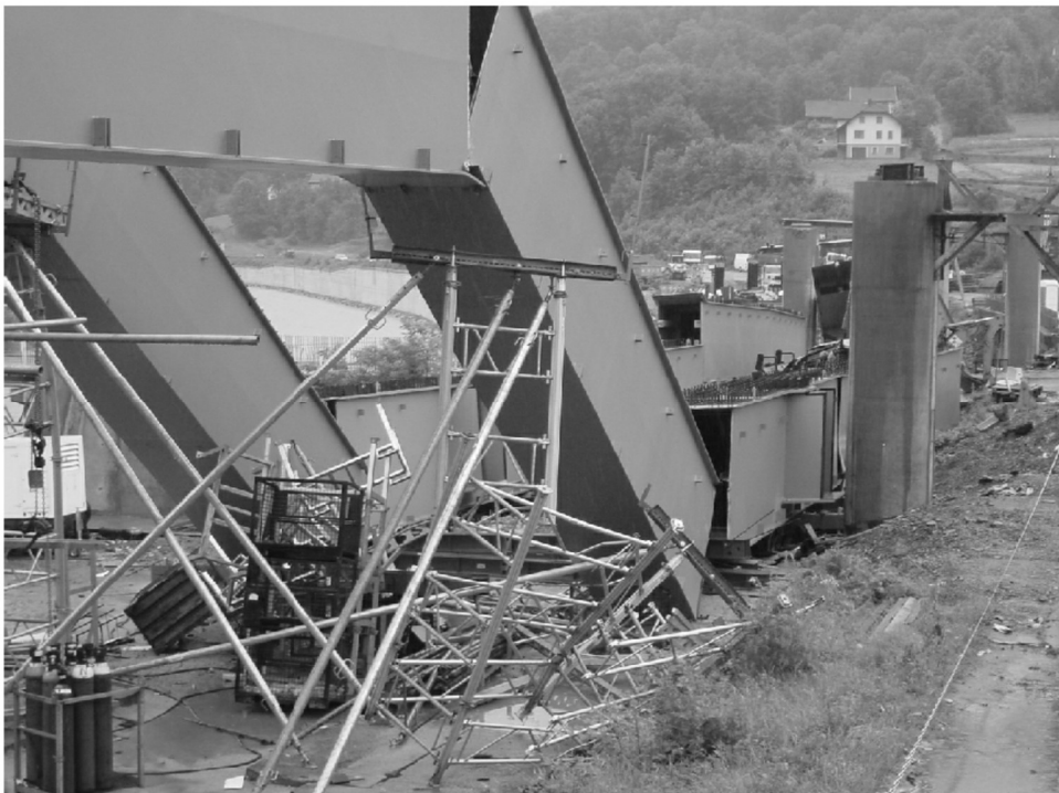
Photo 10. General view of the destroyed viaduct structure in Stróža, (according to Prof.PL, M. ŁAGODA, Lublin University of Technology, Road and Bridge Research Institute, Warsaw 2007)
