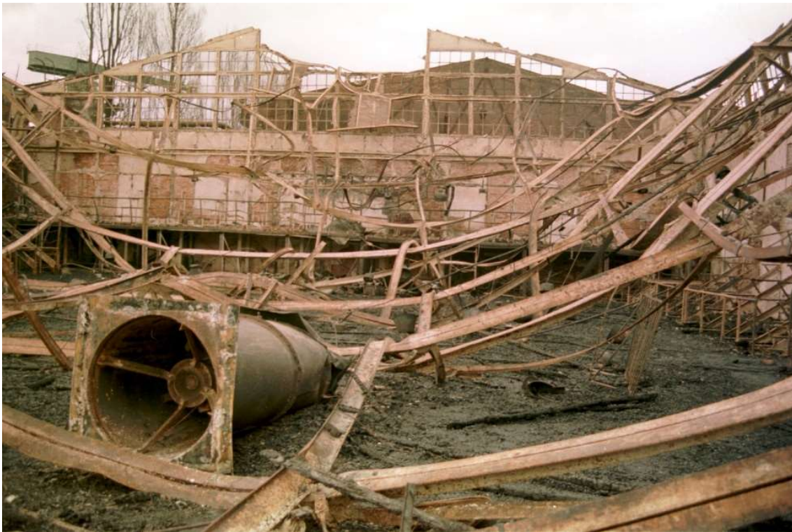
Photo 5. Steel structure of the Gdańsk Shipyard hall after the disaster caused by fire (1994 r.), photo. Maciej Kosycarz/KFP
