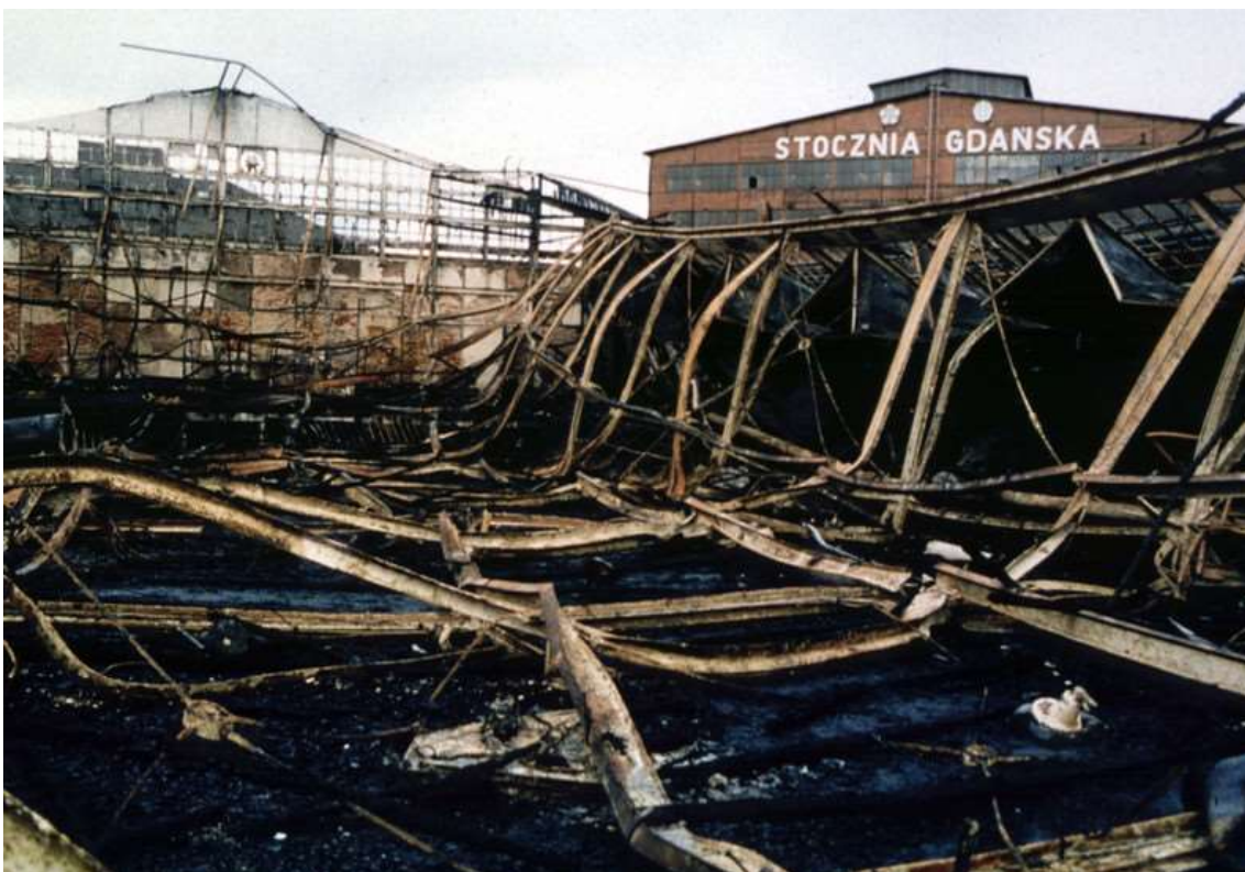
Photo 6. Steel structure of the Gdańsk Shipyard hall after the disaster caused by fire (1994 r.), photo. Maciej Kosycarz/KFP
