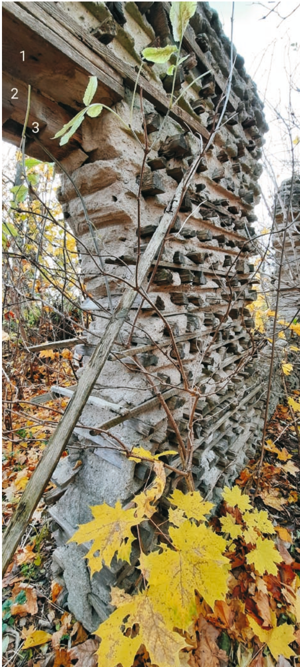
Fig. 10. Wall and carpentry details of the cordwood house in Rydzewo Kolonia: (1) door lintel; (2) door header; (3) mortise; photo: Renata Adamska and Katarzyna Karwowska, 2021
