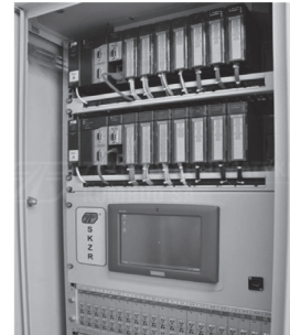
Fig. 10. The cabinet of SKZR-2 system with GE Fanuc PLC controllers and a diagnostic panel [19]
