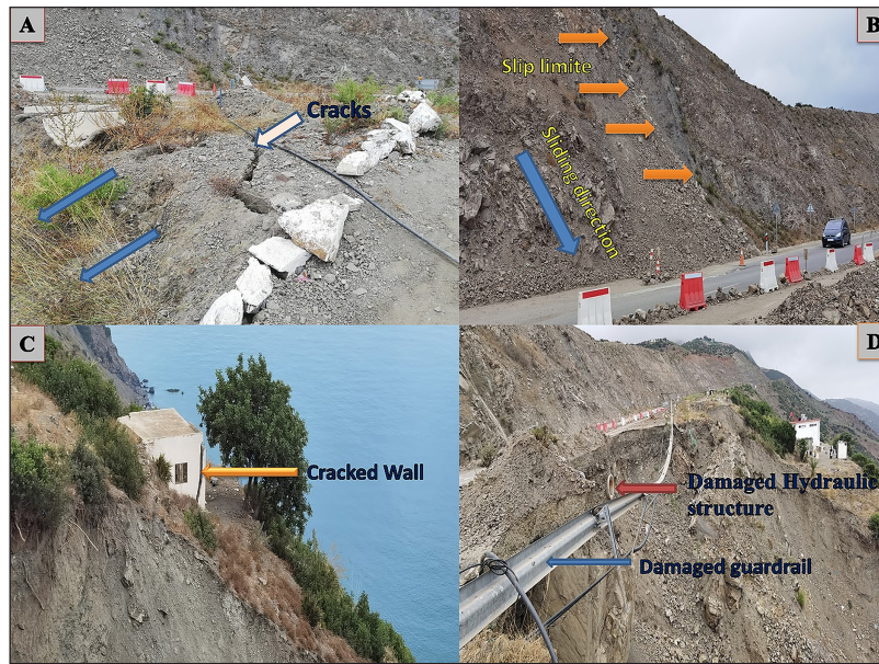
Figure 5. (a) Cracks and subsidence in the road sides, (b) limit and direction of the slide, (c) crack in the wall of a small house, (d) collapse of the roadway and damaged structures
