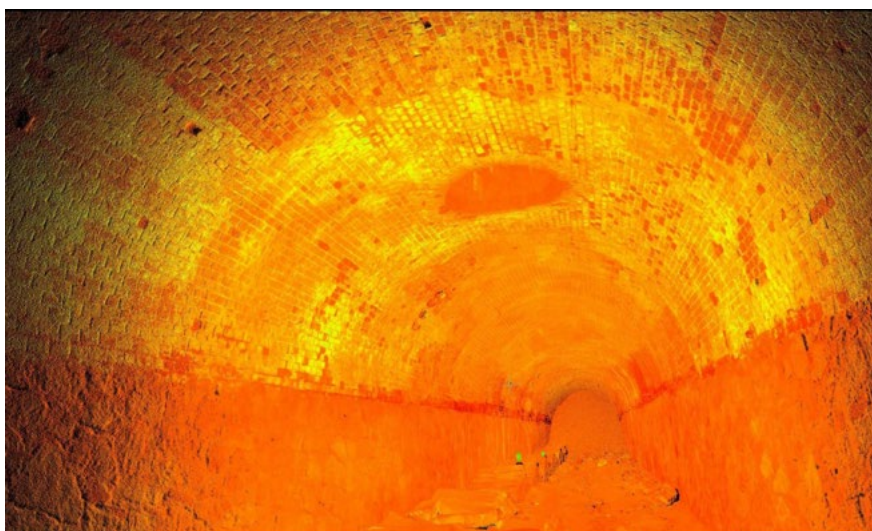
Fig. 7. A 3D view of the interior of the postern generated with the Leica Cyclone software – the authors' own elaboration
