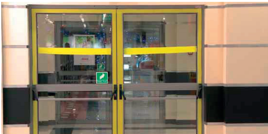
Figure 14. Contrasting marking of glass doors
