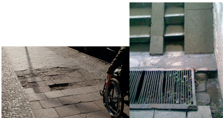
Figure 5 and 6. Examples of inappropriate adaptation of infrastructure to the needs of people with special needs
