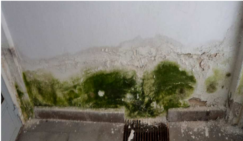
Photo 1. The external building wall with visible biocorrosion on the building of the former UZ canteen
